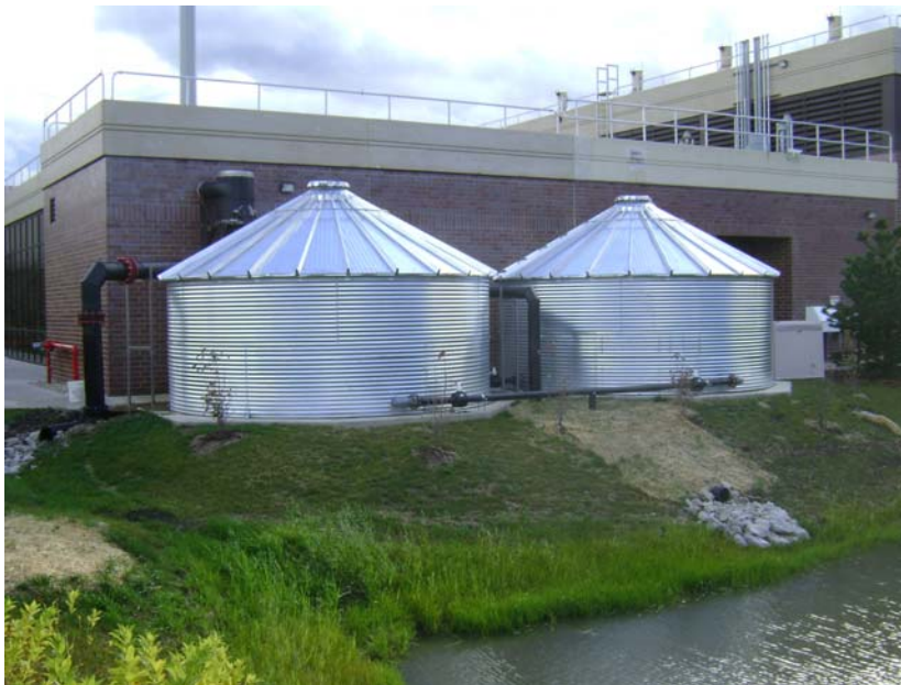
Rainwater Collection System
