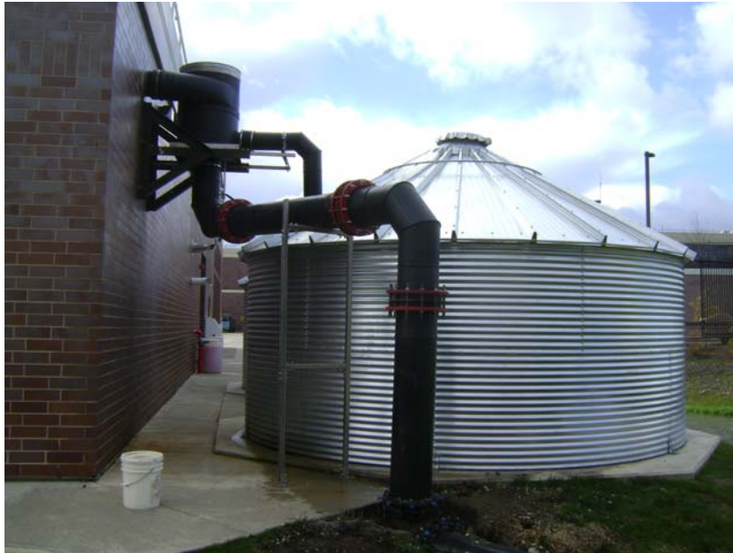
Rainwater Collection Filter & Piping
