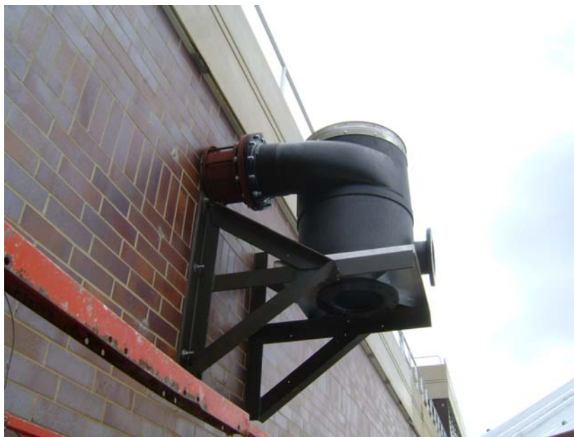
Rainwater Collection System Filter
