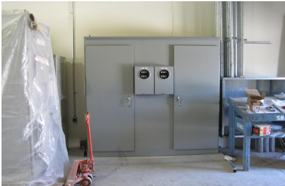
CT Meter Cabinet
