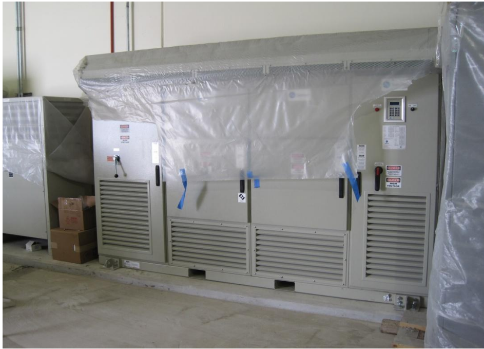
New PV Inverter
