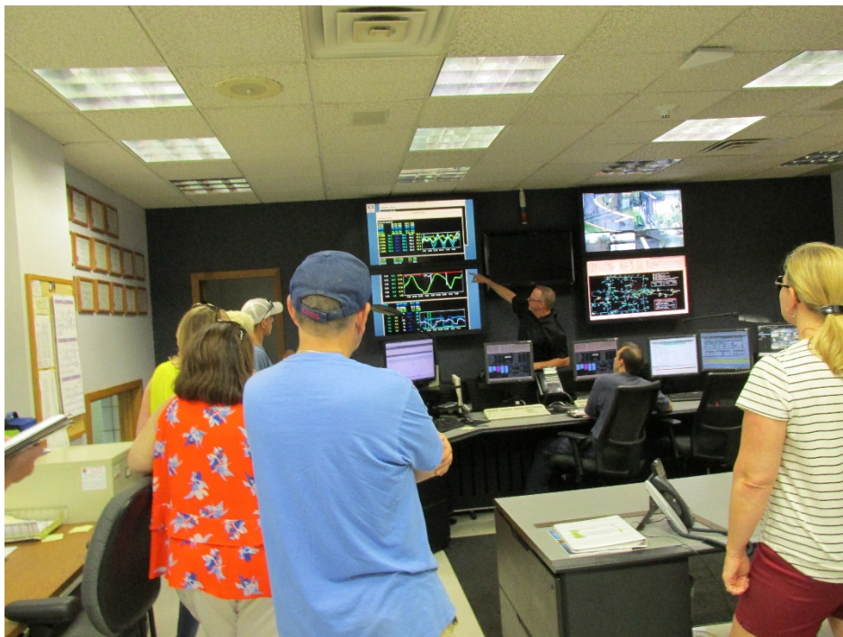
Mike Weed reviewing how the control room operator controls valves, pumps, and tanks from a central location
