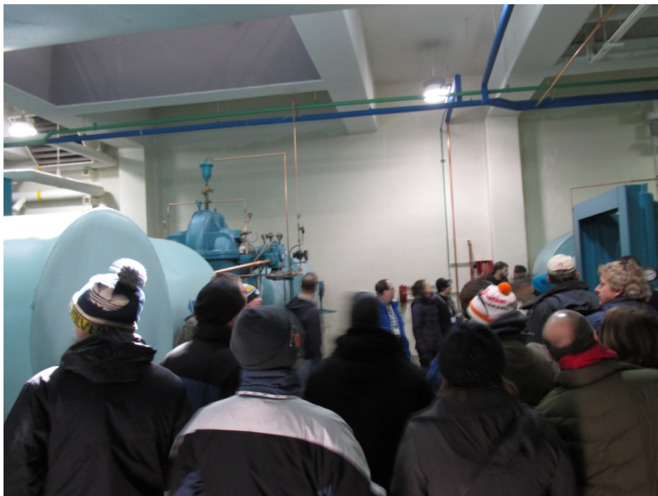
The teachers viewing DWC's large pumps
