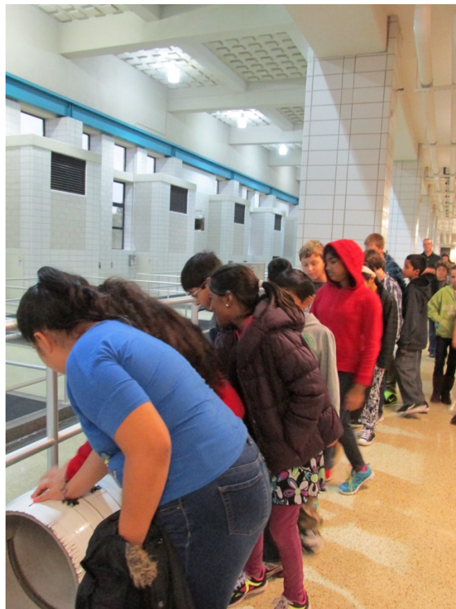
Students had the ability to view and touch the different types of pipes DWC utilizes in the field
